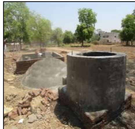
Developed Biogas Based Electricity Plant
