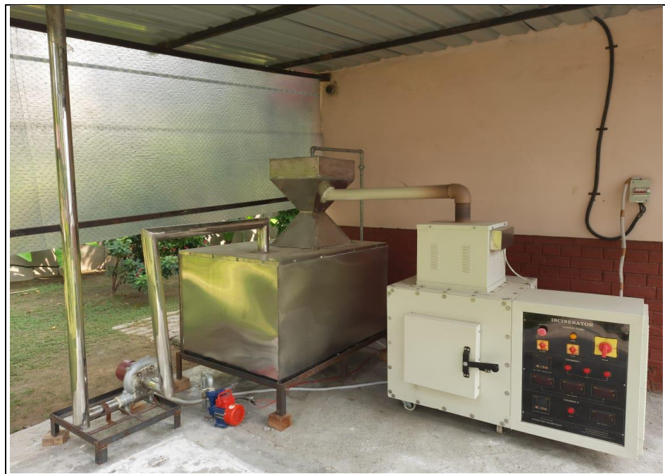
Bio-hazard waste Incinerator
