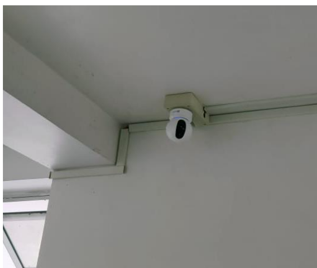
CCTV camera installed in Administrative Building, AAU, Jorhat
