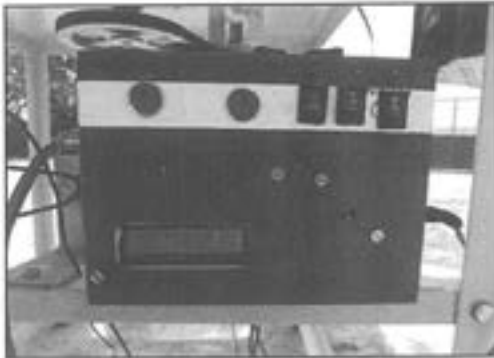
Plate 4.1 Control panel of dual axis tracking system
